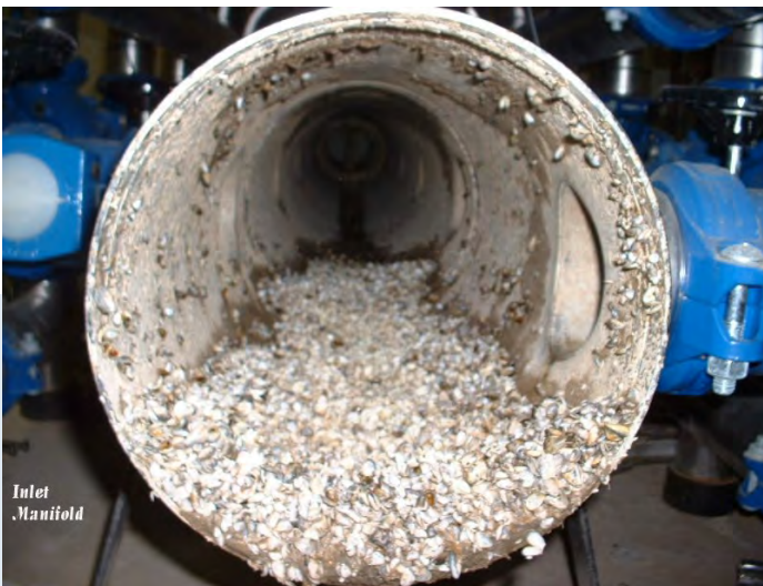
Intake manifold (before filter)
