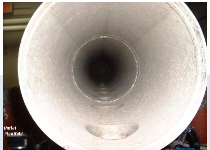
Outlet manifold (after filter)
